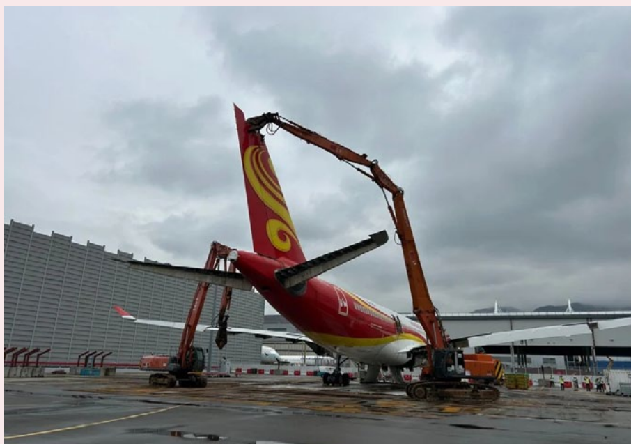
Disassembly of one of the six A330-200 aircraft at Hong Kong International Airport
