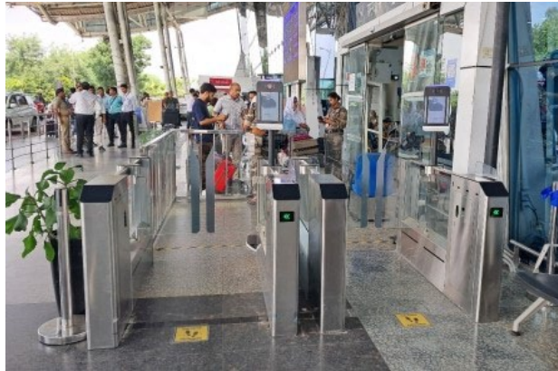
SITA is installing its Smart Path technology across nine Indian airports in a partnership with AAI © SITA
