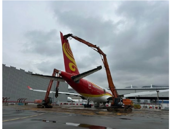
Disassembly of one of the six A330-200 aircraft at Hong Kong International Airport © AerFin
