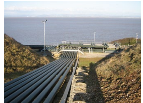
Exolum will invest £4.5 million in a new SAF blending facility in Redcliffe Bay in south-west England © Exolum
