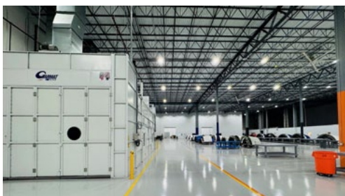
The expanded facility features newly installed, state-of-the-art equipment, including a 40-ft heating oven, 40-ft paint booth, and a 24-by-24-ft sanding booth
